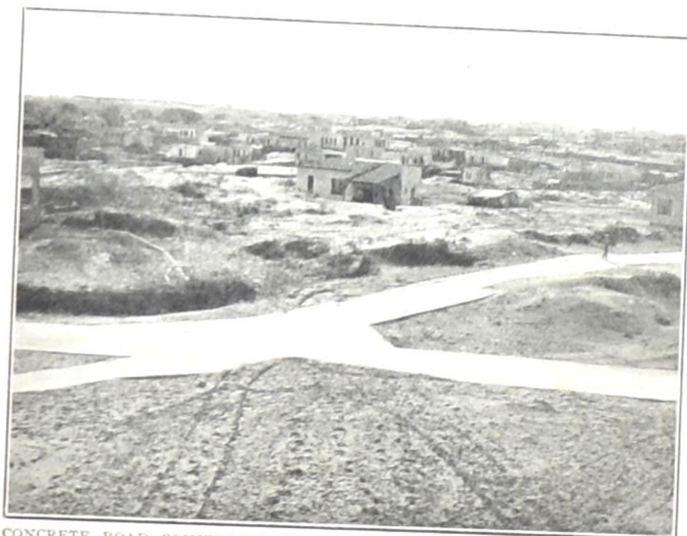
CONCRETE ROAD CONSTRUCTION ON SAND AT TEL AVIV, CARRIED OUT BY THE JEWISH CO-OPERATIVE LABOUR ASSOCIATION WITH AMERICAN AND ENGLISH CONCRETE MIXERS.
