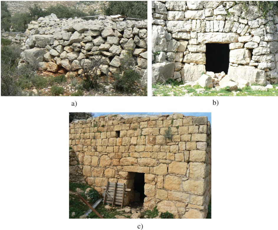
Figure 10. Photographs of the three categories of watchtowers in the study area, showing especially the texture of the stonework and the dimensions of the stones in each; the distinctive styles are most evident in the lower courses and around the door openings: a) a rounded stone heap, b) a corbelled stone watchtower, and c) a quadrilateral dressed ashlar stone watchtower (color figure available online).
