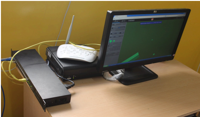
Figure 3: Internet connection in the computer club
