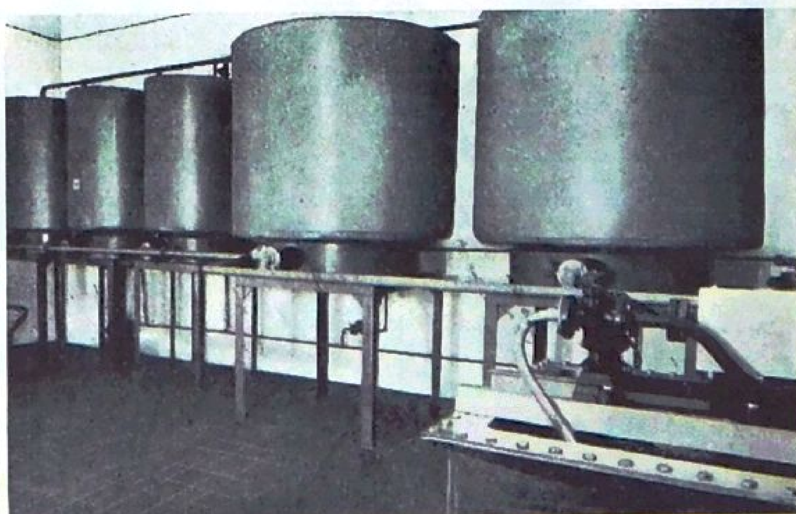
Oil Storage Tanks
