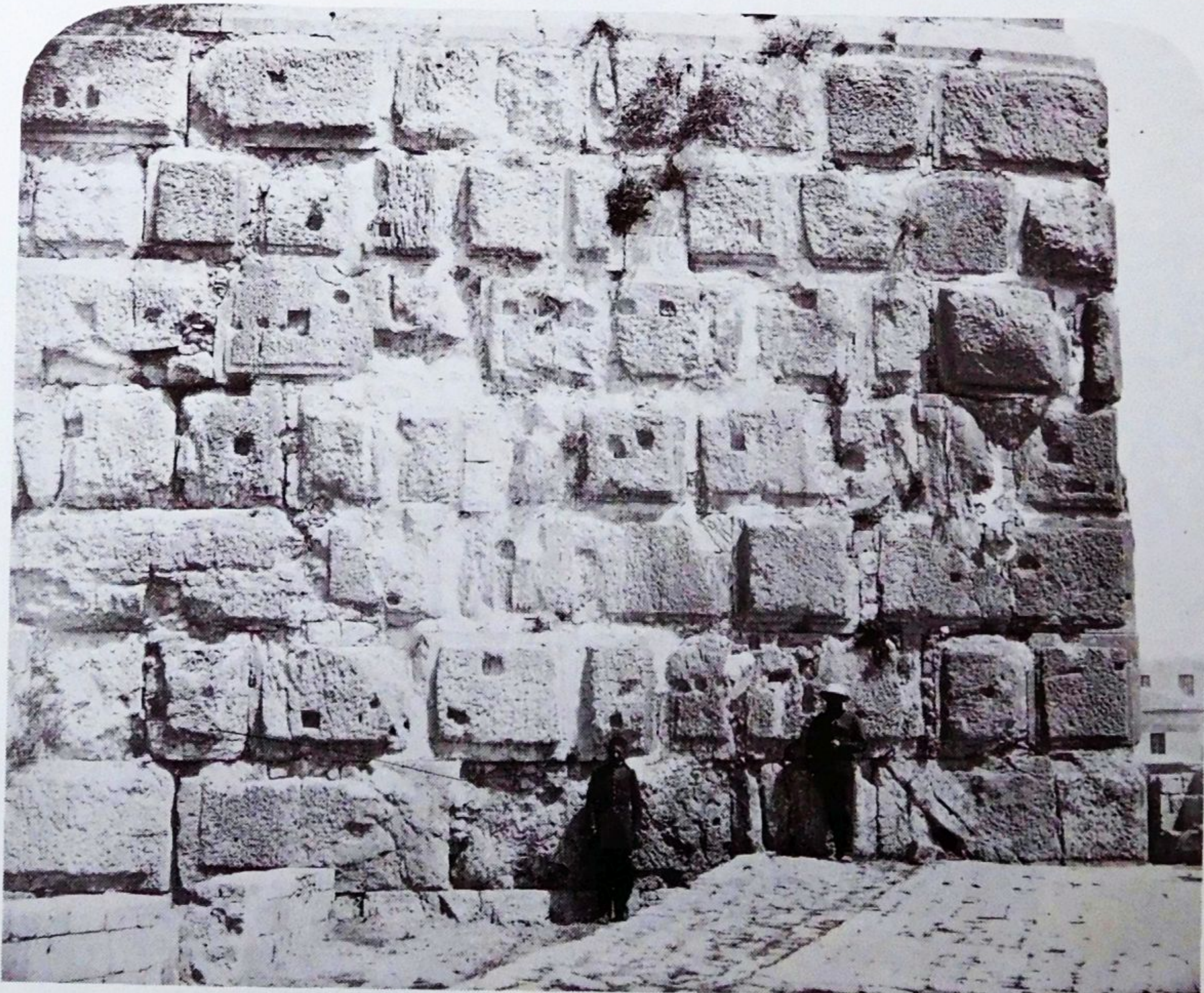
21b. DETAIL OF LOWER PART OF THE N. E. TOWER OF CITADEL
